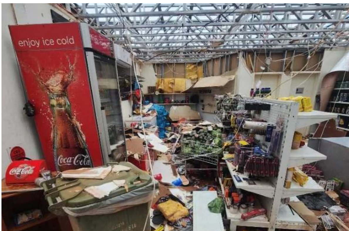
Figure 2: Devastation incurred at Pardoo Station. (ABC News: Pardoo Roadhouse and Tavern).
