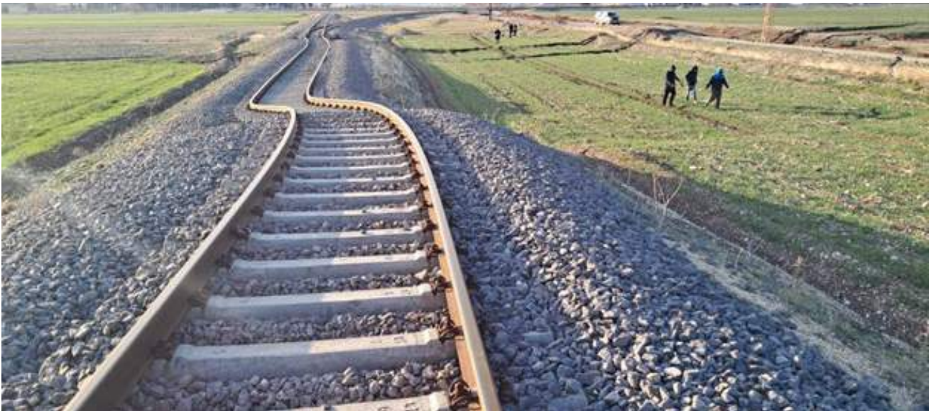
Figure 9. Surface rupture at Hassa (located near Iskenderun in Figure 2), showing left-lateral offset of the centreline of the road. Source: Ozdemir Alpay (2023).
