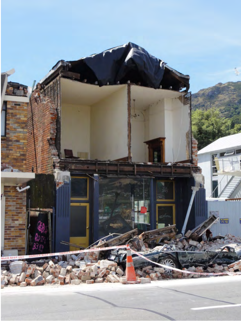
Figure 2. Failure of gable end and upper storey facade. Note the unfortunately parked car on the street below.
