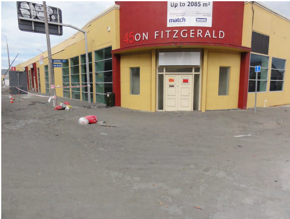
Figure 10. Liquefaction around shop entrance on city cordon. Note also cracking to parapets.
