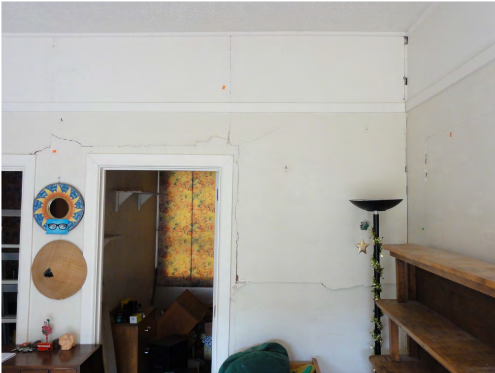
Figure 4. Extensive internal cracking of timber framed home.
