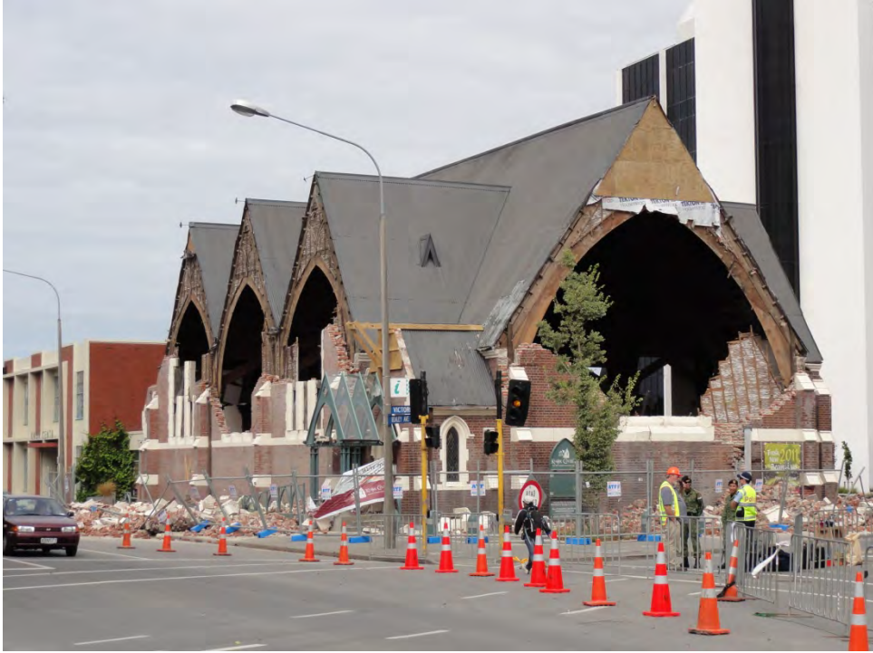
Figure 7. Loss of gables on the Presbyterian Church.
