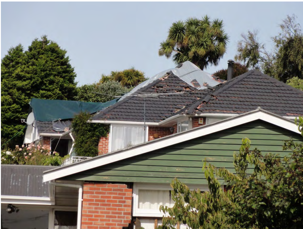
Figure 6. Damage to newer tiled roof.
