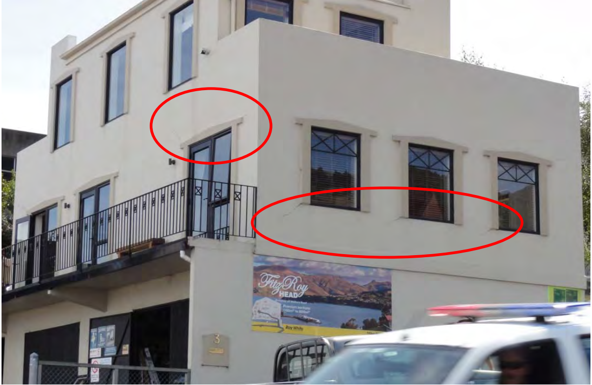
Figure 3. Cracking from edges of door and window frames, but no failure of newer buildings.
