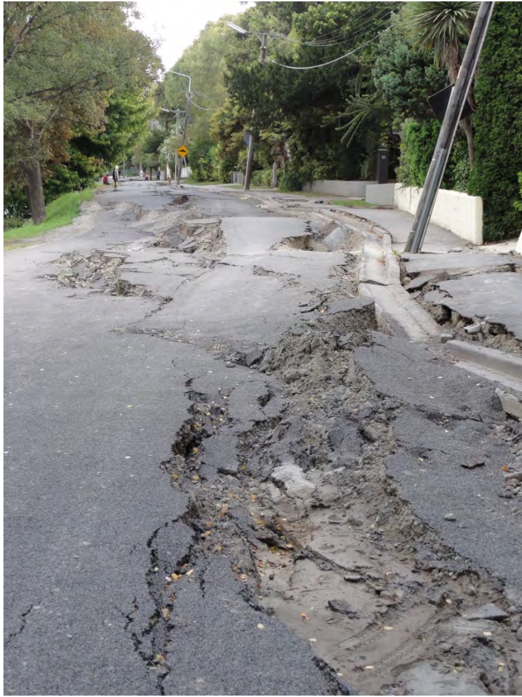
Figure 8. Damage to road along Avon River.
