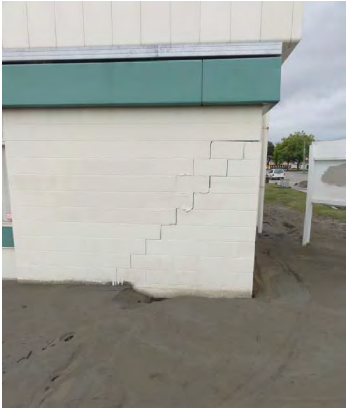
Figure 7. Cracking of building caused by liquefaction.
