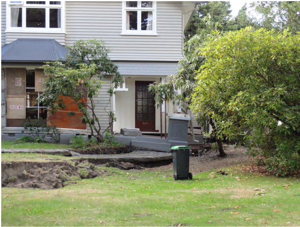
Figure 6. Undermining of foundation through lateral spreading.
