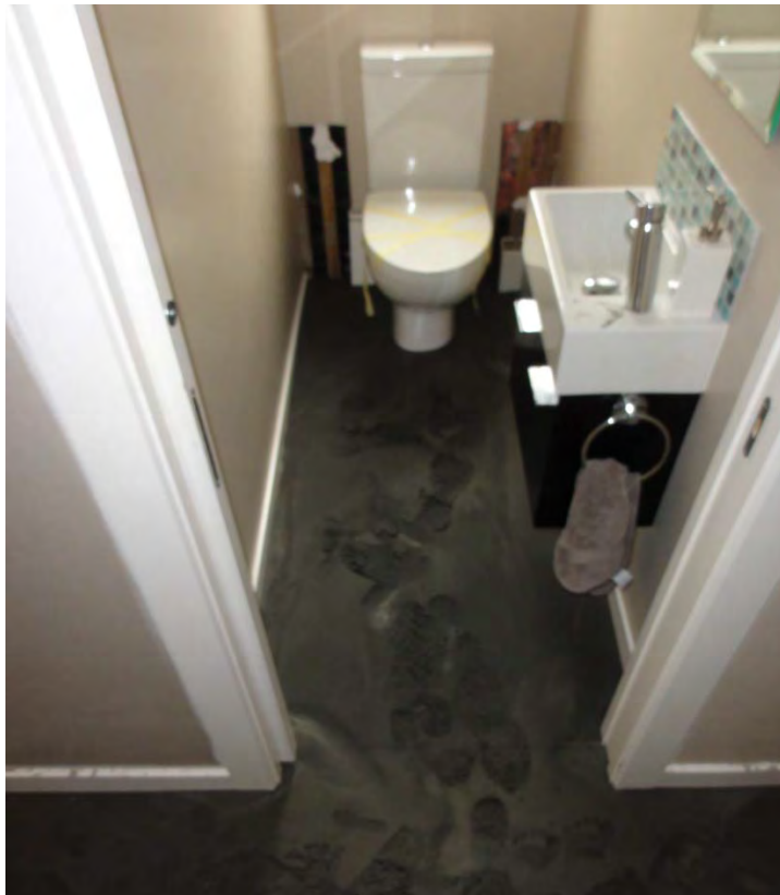
Figure 1. Damage to the living room (upper image) and bathroom (lower image) of a home in Halswell.
