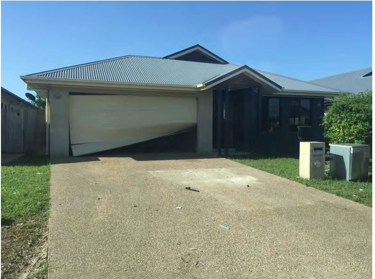
Figure 2: Roller doors in Eastern Idalia potentially damaged by an electrical short. High flow flood waters were ruled out as a cause based on lack of debris and vegetation.
