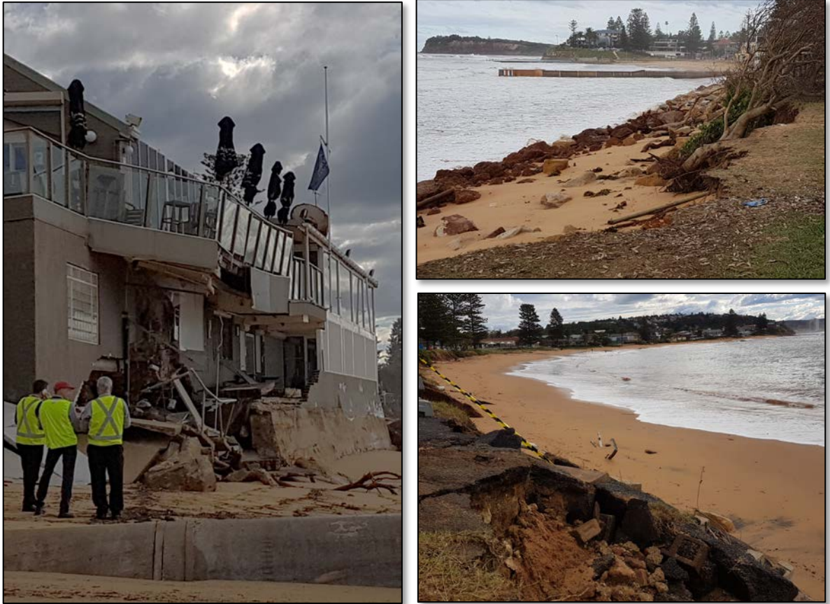
Figure 2 (clockwise from left) severe structural damage to the Collaroy Beach Club; beach lowering at South Narrabeen (sewage pipe is usually buried under beach); cliff failure and car park damage at Fisherman's Beach.
